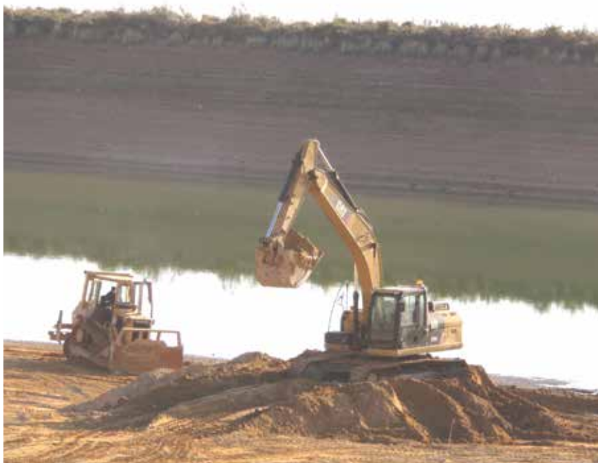
At the end of last summer, the dams were cleaned and silt removed. Underwater mountains of rubble were found.
